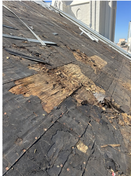
Left, rotten material is revealed once the old metal roof was removed.
